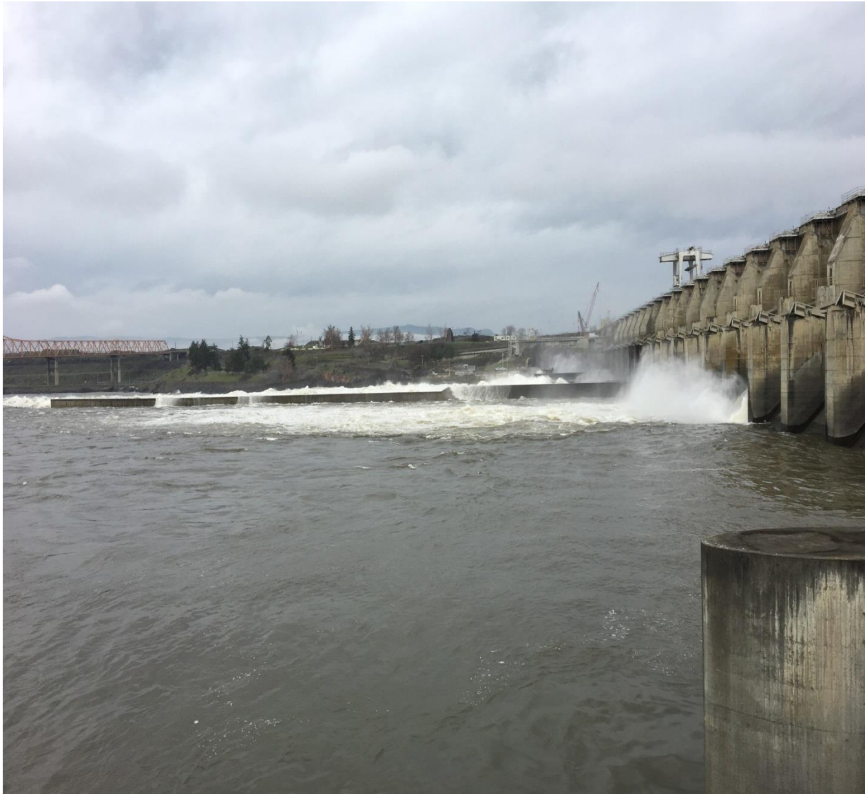
High spill overtopping wall.
